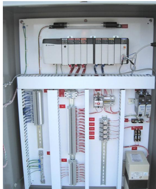
Photo of small PLC system cabinet.
